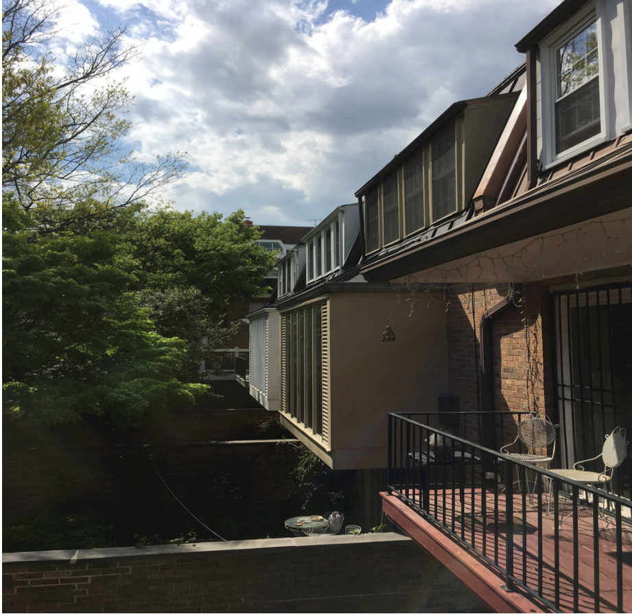
Photo 6: Back view of immediate neighbors bump outs. These bump outs extend out beyond what applicant's proposed bump out would be. Proposed bump out would bring applicant's back of house even with brick rear walls.
